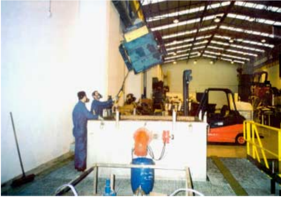
Workers wearing protective clothing while handling a PCB transformer.
